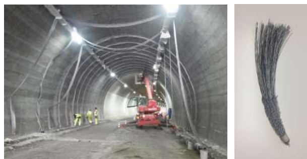
Figure 15. Systematic lining reinforcement by Steel net and detailing of connector (SFIX G 12)
