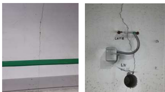
Figure 11. Monitored vertical cracks
