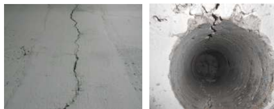
Figure 13. a) Longitudinal crack, b) checked by coring
