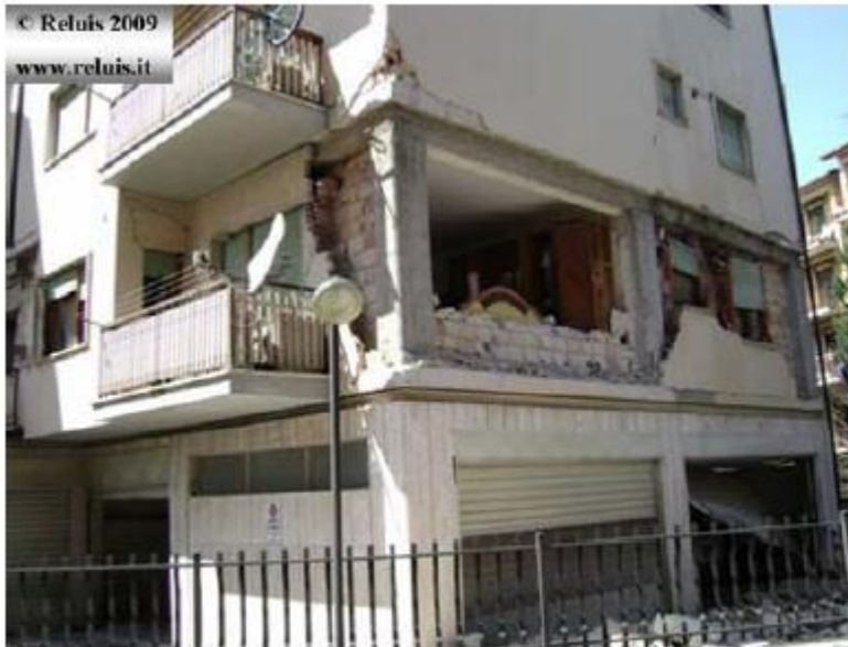
Reinforced concrete building placed in Via XX Settembre – L'Aquila Total and partial ejecting of corner infills at first level.
