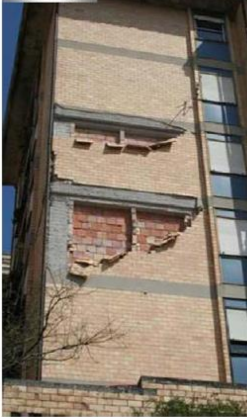
Infills damage Internal infill is made up of clay blocks
